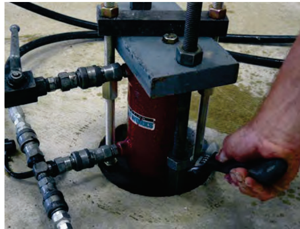
Figure 2.80 Pier load locked off by tightening nuts on top of pier cap
