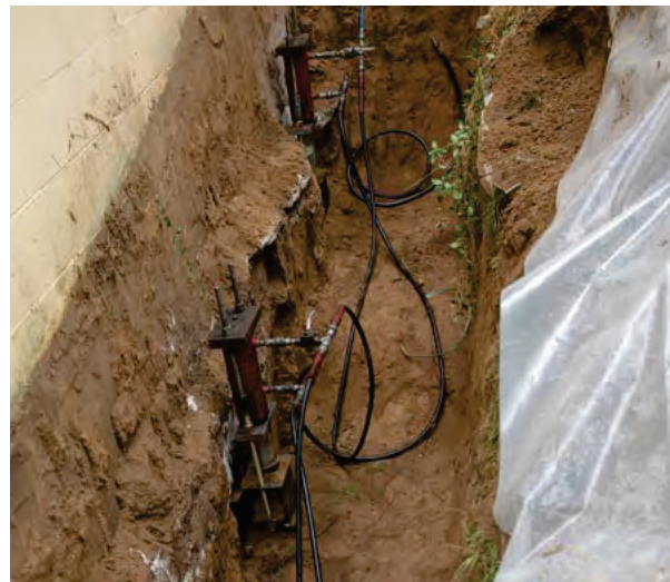
Figure 2.41 Hydraulic system connected to provide uniform application of load
