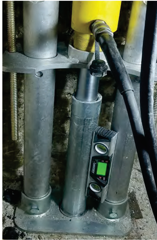
Figure 2.53 Check alignment of drive stand and starter section
